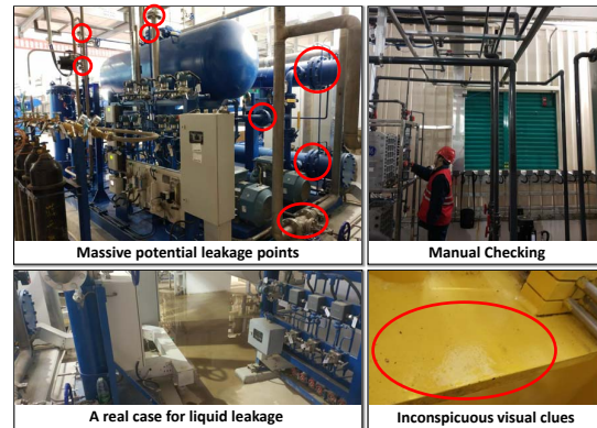
Fig. 1. Liquid leakage problems in modern factories.
